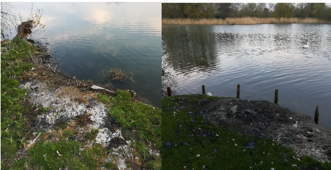
Figure 7 Two examples of Bird damage to the banks
